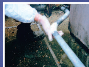
Fast-setting, moisture cured ThistleWrap Pipe Repair Tape used to repair a leaking pipe.
